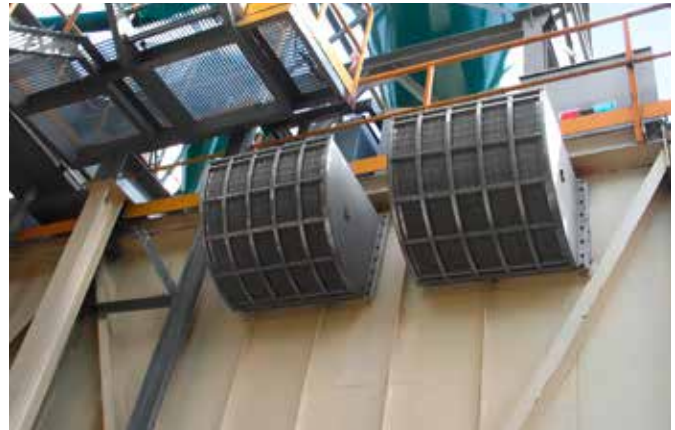
Explosion venting of a chip bunker using the Q-Box to protect the surrounding infrastructure.
