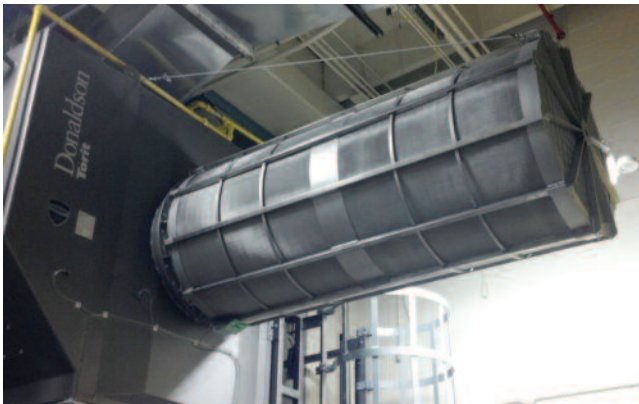
Indoor venting system
